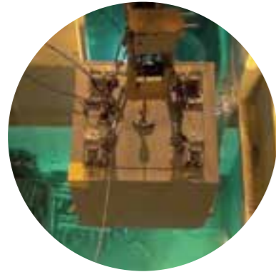
José Cabrera NPP dismantling: Design and manufacturing of special shielded transport bells.
